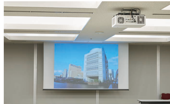
▲ The PT-MZ780 was installed in the rental conference room to increase the brightness so that meetings could be held without dimming the lighting, as in the main hall.
