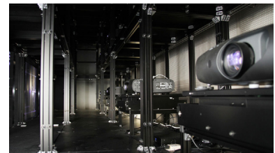
The PT-RZ475 projectors installed inside the cabinet.
