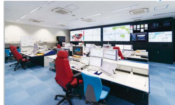
▲ Since the depth of the multi-screen system is shallow, the control room space can be effectively used.
