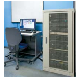
The images displayed on the facility displays are centrally managed using a management server and confirmation monitor.
