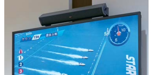
▲ Once the races begin, the live images are displayed on one entire screen. WS-LA100 line array speakers are installed on the upper part of the displays.
