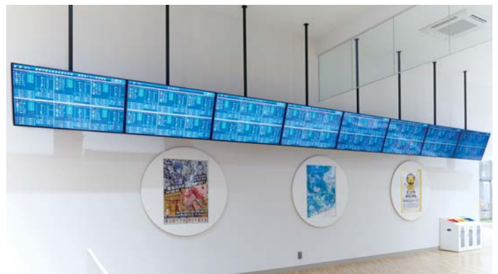
▲ Eight TH-55LFE8 models are installed horizontally along the wall nearby the entrance. Information, such as the betting odds and records from eight different venues, is displayed in real-time.
