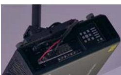
▲ Establishing a network of projectors within the facility with LAN cables
