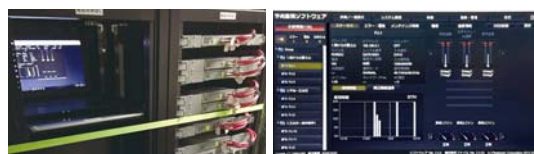
▲ A computer equipped with the Early Warning Software has been installed on the rack inside the control room.
