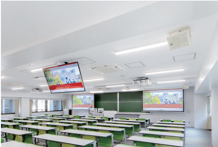
▲ A medium-sized classroom. A total of four RAMSA Near Field Speaker Series 16-cm 2-Way Speaker WS-NF055 units are installed on the front, rear, left, and right of the ceiling.
