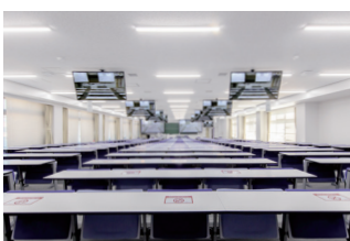
▲ The Large Lecture Theater in Seishinkan also had LCD displays and LCD projectors installed. For projectors, two 13,000-lm PT-MZ13KJL units were used.
