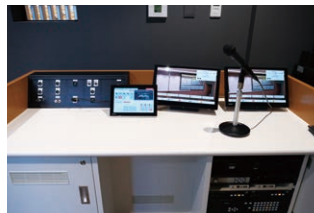
▲ Table for operating the AV equipment in the large lecture hall. Enables centralized control of audio and visual functions, including switching between the two and sending video and images of the classes using the HD Visual Communication System.
