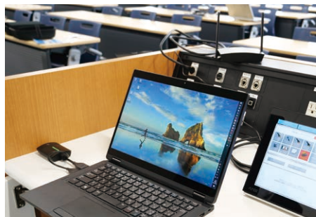
◀ The PressIT Wireless Presentation System installed in the training room. A PC screen can be shared on a projector and display, simply by connecting it to a PC and pressing a button. Compact and portable, it can easily be taken to different classrooms.
