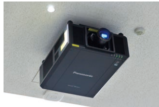
▲ PT-RZ21K 3-Chip DLP® Laser Projector installed in the ceiling of the large lecture hall
