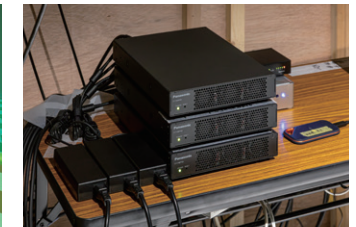
▲ ET-FMP50 installed in the backstage area.
