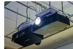
▲ PT-MZ20K and PT-MZ17K units installed throughout the Yokai Hyakki Yako zone.
