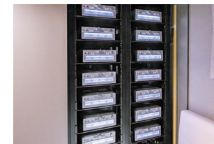
▲ Equipment rack housing 14 Technics amplifiers
