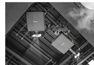
▲ Light-blocking hoods mounted on each lens to isolate projection areas, preventing visual overlap within the circular theater
