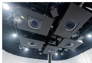
▲ Projectors, speakers and vortex rings installed across the ceiling of Zone 4
