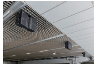
▲ A row of 11 pairs of speakers are suspended from the roof to create an immersive acoustic space
