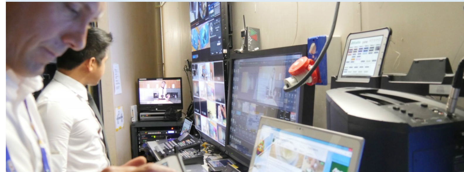
The broadcast control room at Etihad Pavilion
